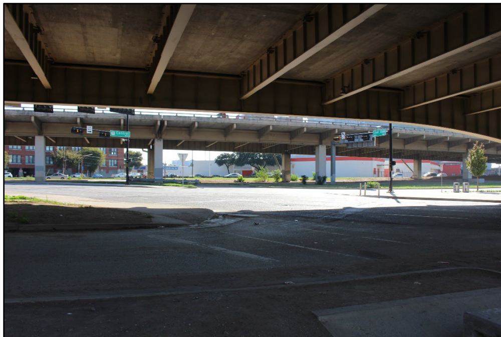
Photo 14 – Looking southeast at the existing intersection between the existing I-345 facility and Live Oak St.
