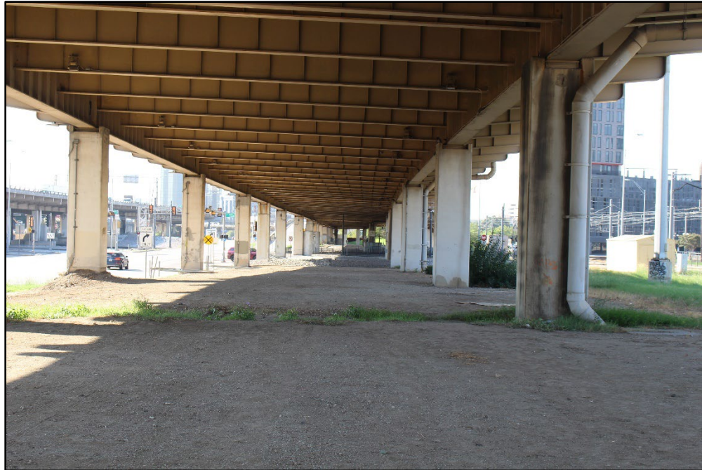
Photo 11 – Looking south at the existing terrain underneath the I-345 mainlanes which is rough in some areas, making it difficult to walk or bike across/along the facility.
